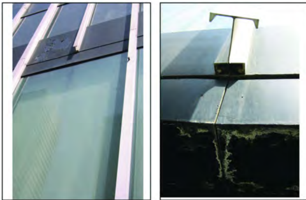
Middle left to right; Telus building damage and finish failure on the west side of the building;
